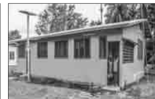
Piano Health Center getting a facelift to its maternity ward, with support from the Regional Member for Bougainville.
